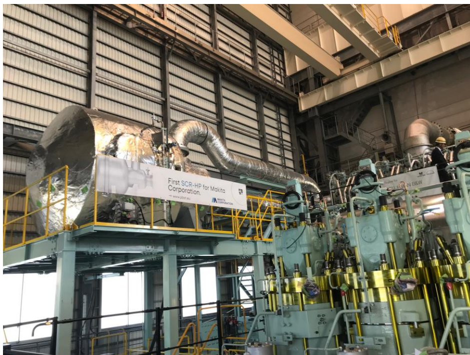
SCR-HP cluster 3 mounted on the engine during engine shop test.
